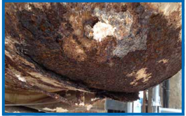
Corroded vessel: Corrosion Under Insulation (CUI)
