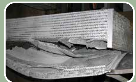
Cross section through the bulged region of an aluminum plate fin heat exchanger.
