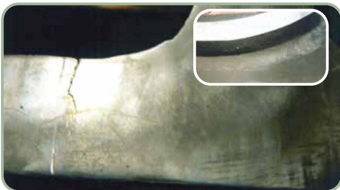
ID cracks adjacent to repair welds
