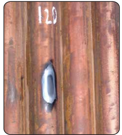
Polished FMR site on a boiler tube
